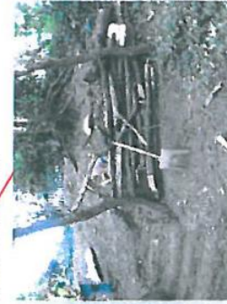
Section 4. Digger access was not possible so it was cleaned by hand. There are a number of trees disrupting access which should be removed, as well as the trees within 2m of the section. Trees/scrub immediately downslope can be retained.
