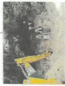
Opening up the lower part of Section 3 using a digger. The upper part of the section is obscured by trees and scrub which should be cleared periodically, as should the area around the section to improve access.
